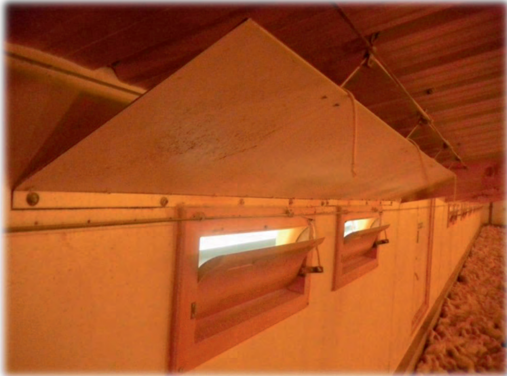
Figure 22 shows a deflector above an inlet - Image courtesy of Mike Czarick,
