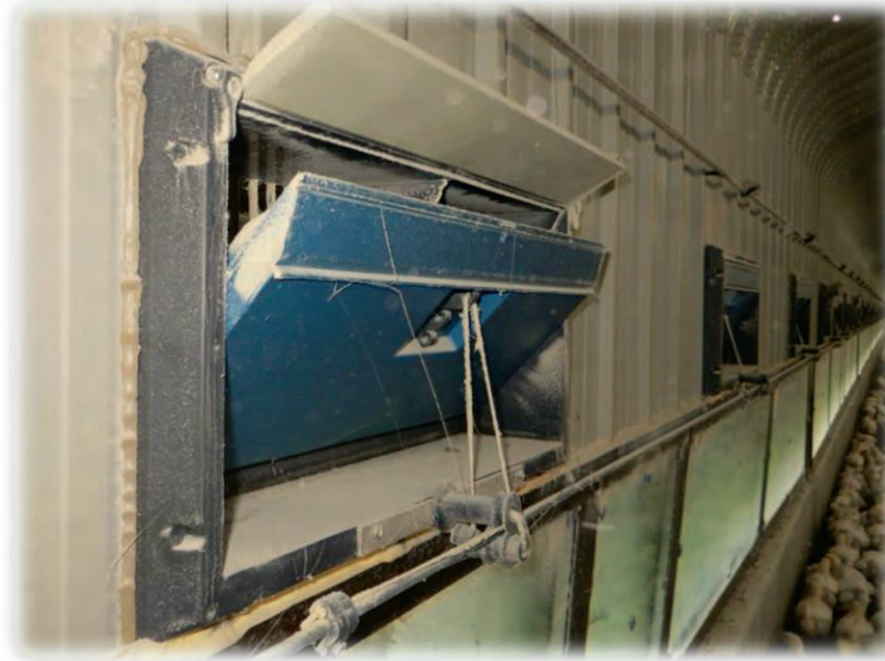
Figure 23 Recessed inlet at a farm in Devon (it also has a small deflector ramp to guide air up towards the ceiling)
