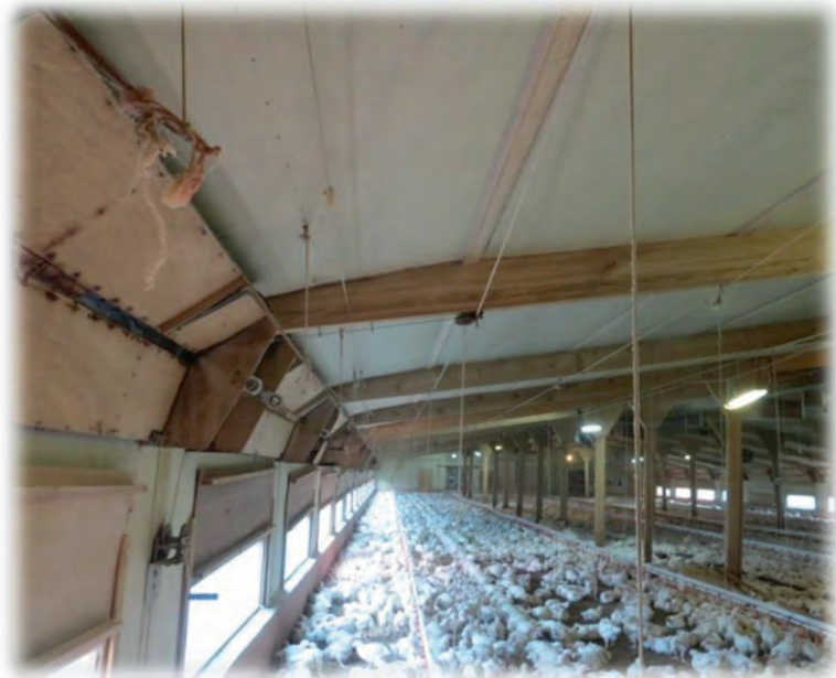
Figure 45 Shows the inlets at Farm B
