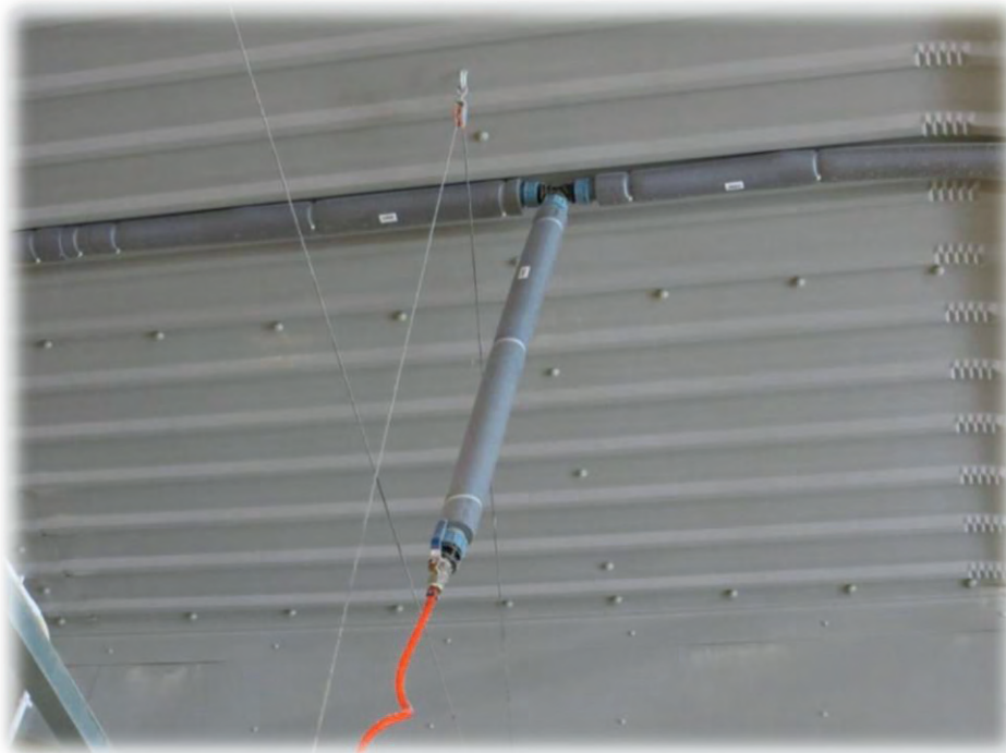
Figure 12 Example of insulated water pipe on a farm I visited in Devon in the UK
