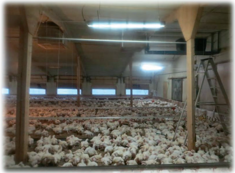
Figure 21 shows a fluorescent light which is facing the wrong way, potentially allowing air coming in through the inlets to hit the light and fall to the litter
