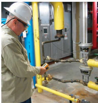
Testing the steam trap to see whether the trap has failed open and is wasting steam.
