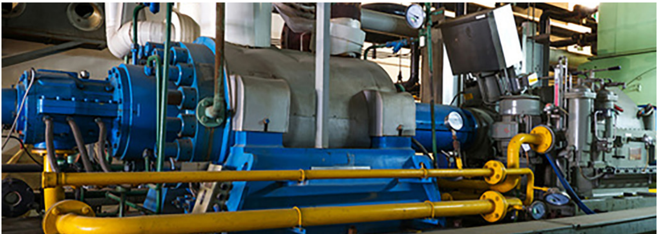
Fig. 1: Boiler systems provide the thermal energy required for numerous processes in power generation, air conditioning in buildings and the chemical industry.
