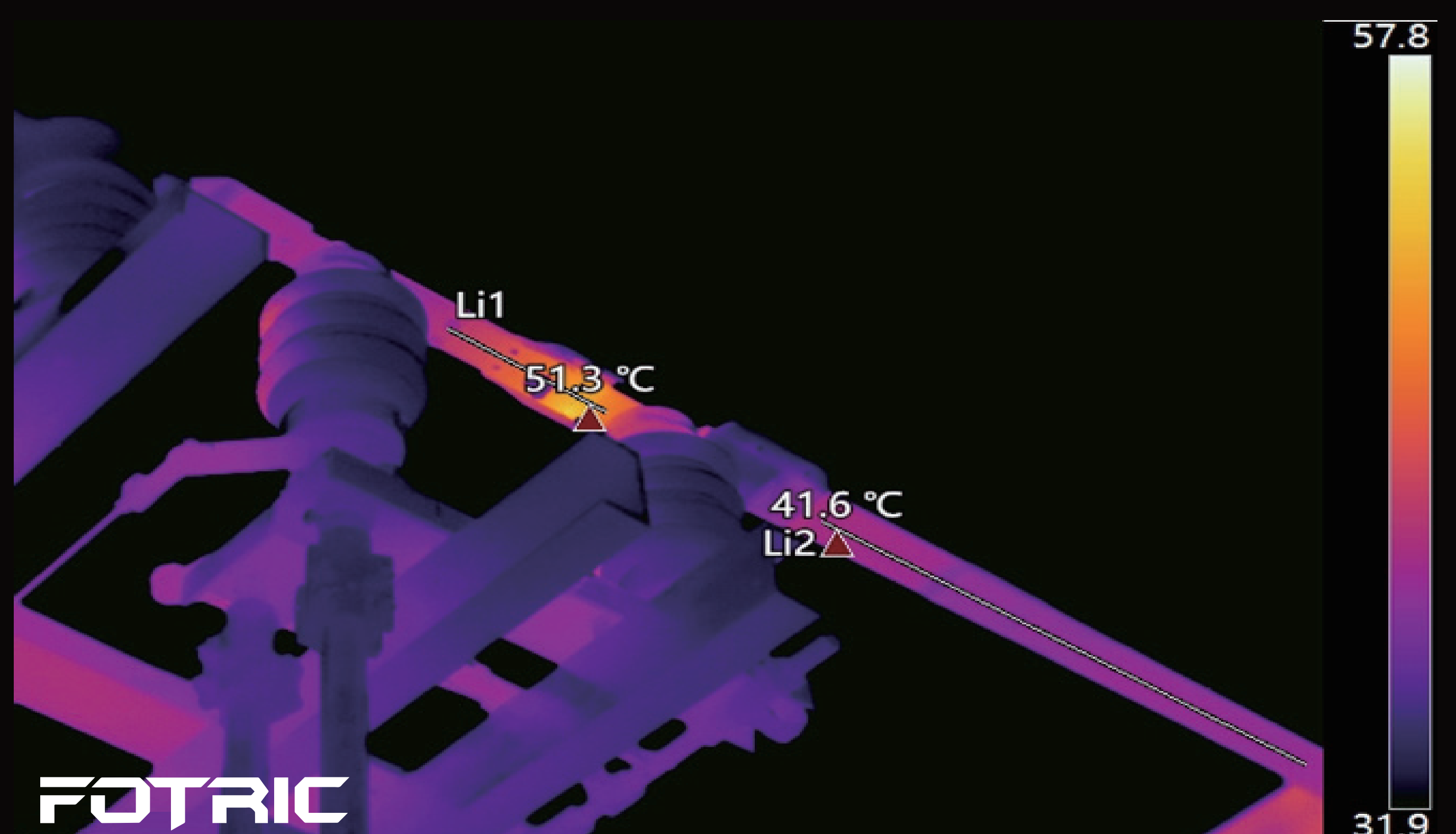
FOTRIC Heat anomaly of an isolating switch in substation
